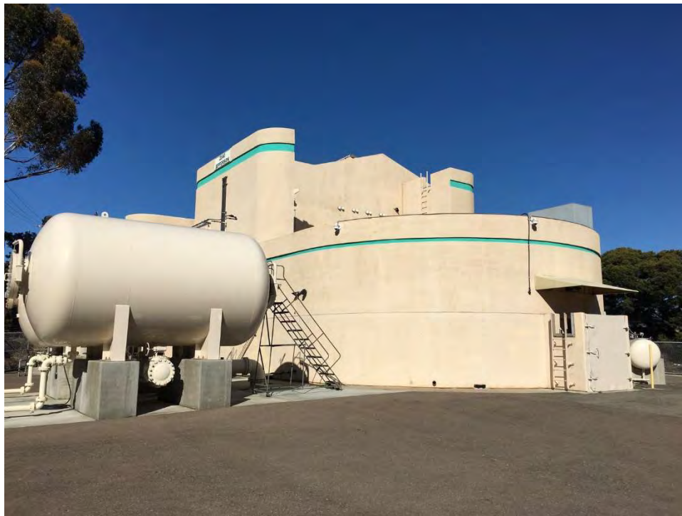
Buena Vista Pump Station
