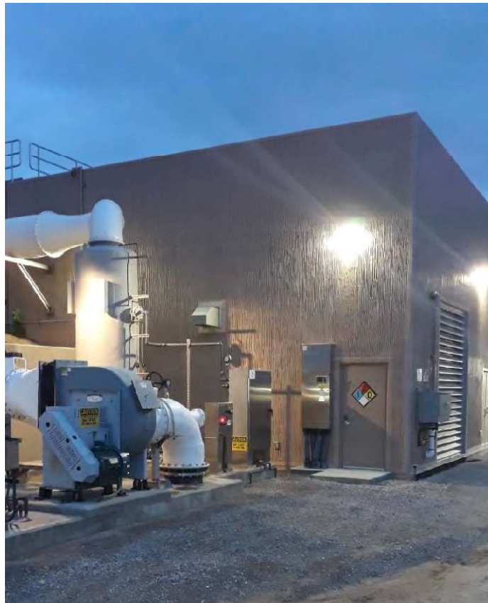
Agua Hedionda Lift Station
