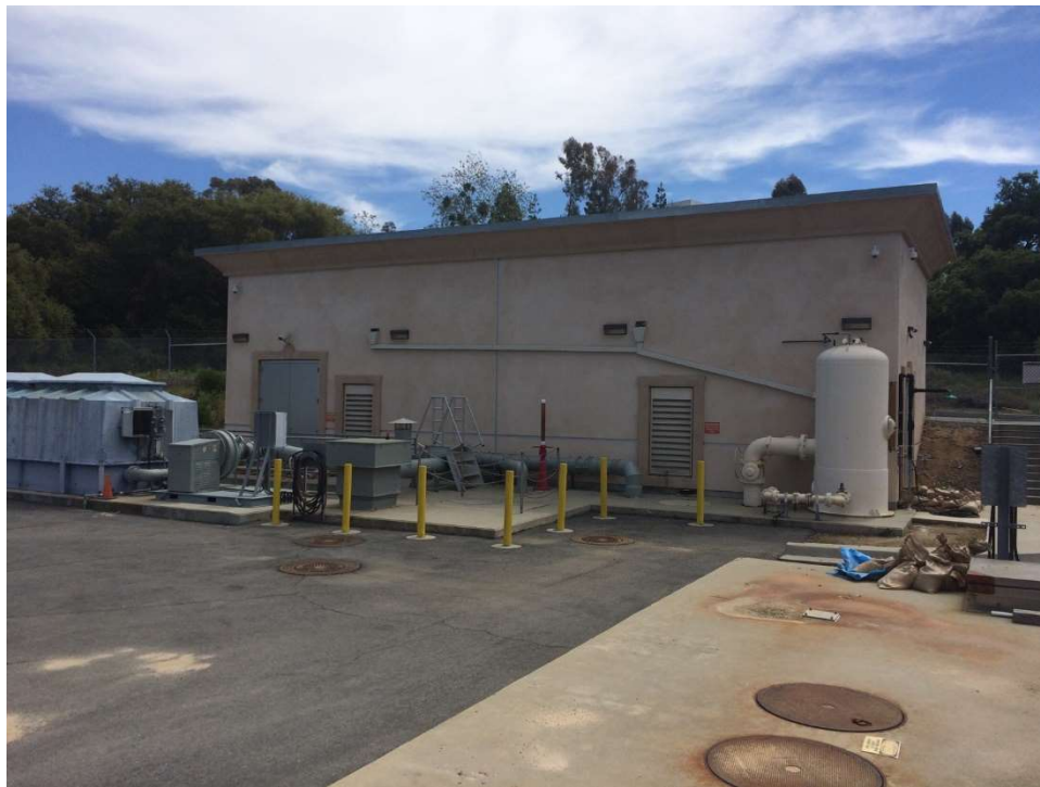
Buena Creek Pump Station
