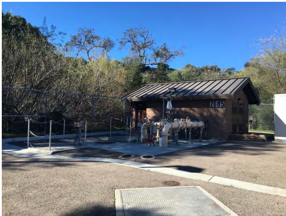
Raceway Basin Pump Station
