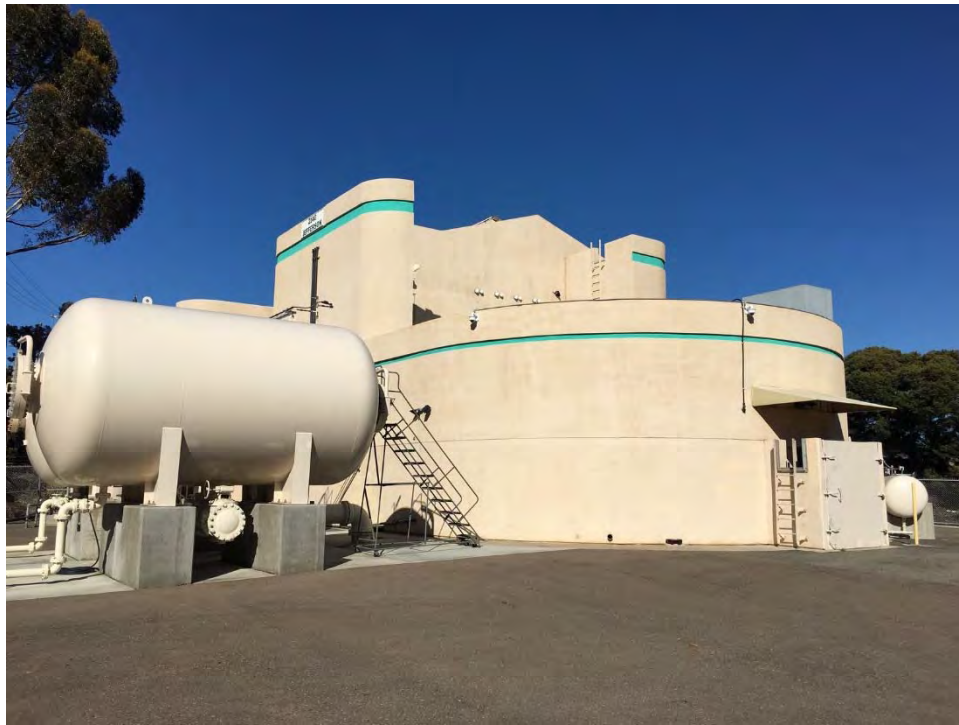
Buena Vista Pump Station
